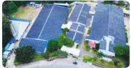
Solar rooftop panels at the Hela Mawathagama manufacturing facility
